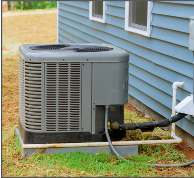
HVAC Example (Split System)
